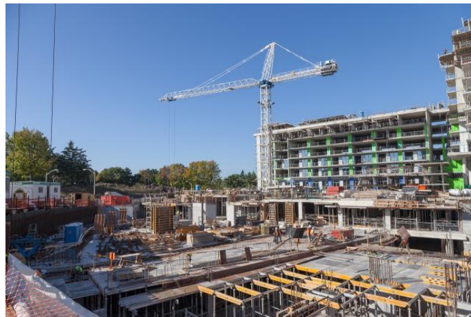
Fifth on the Park soon to rise above grade, image by Jack Landau
