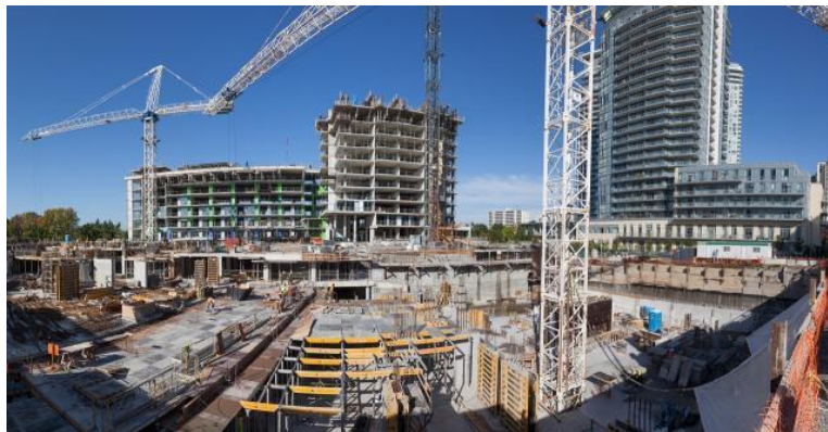
Panoramic view of construction at Emerald City's Block B, image by Jack Landau
